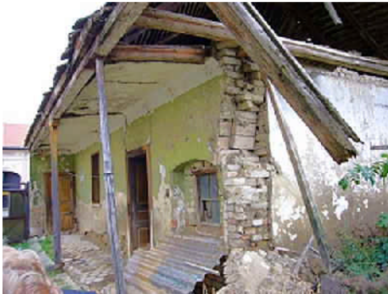
Picture 16 – A very dilapidated house in the Hospital Lane in 2005.
